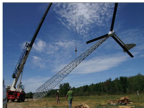
A Bergey Excel 10kW wind turbine installed at Cross Island Farm, NY
