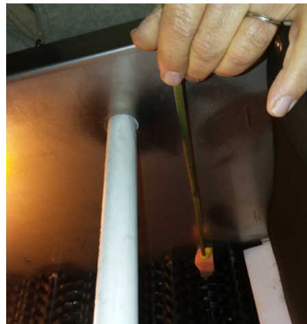
Homemade long-handle scrub sponge can be used to clean dried debris from wall.
